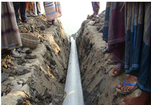
Photo-1 : People fitting pipe by cutting new embankment to get salt water inside Jaliakhali, Gabura (on 16 March'11)
