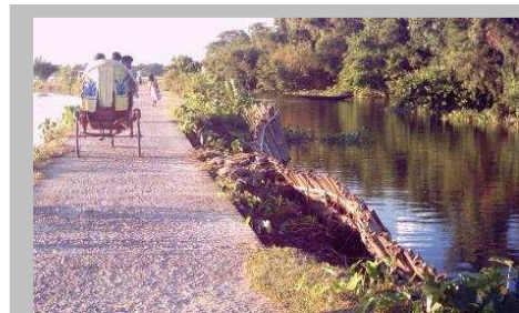
Road embankment eroded by floods Photo: Sunamganj Community-Based Resource Management Project
